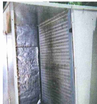
Inner view of a dirty air and heating unit that needs cleaning.
